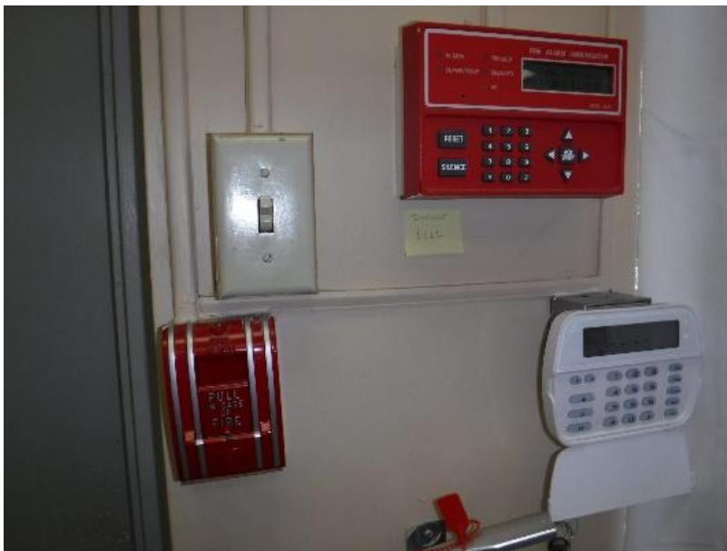
Annunciator Panel and Pull Station
