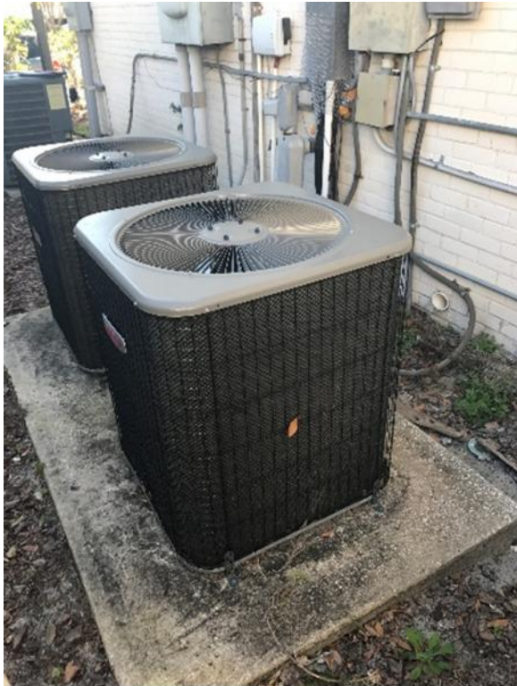
(2) 5 Ton Condensing Units
