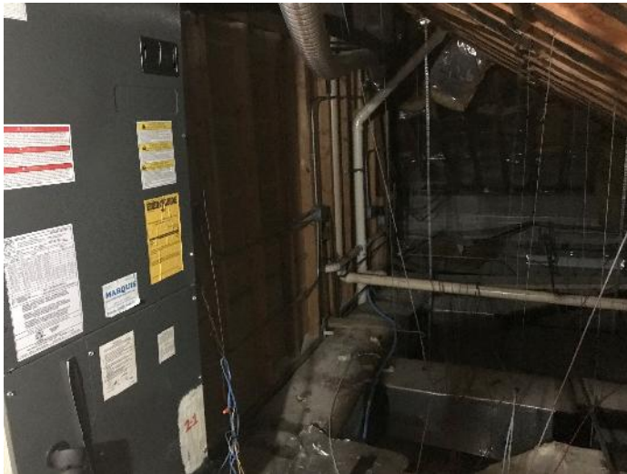
3.5 Ton Air Handling Unit (AHU-2.1)
