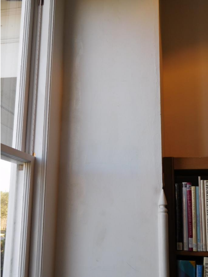
Adult Reading Room wood window system; note water damage
