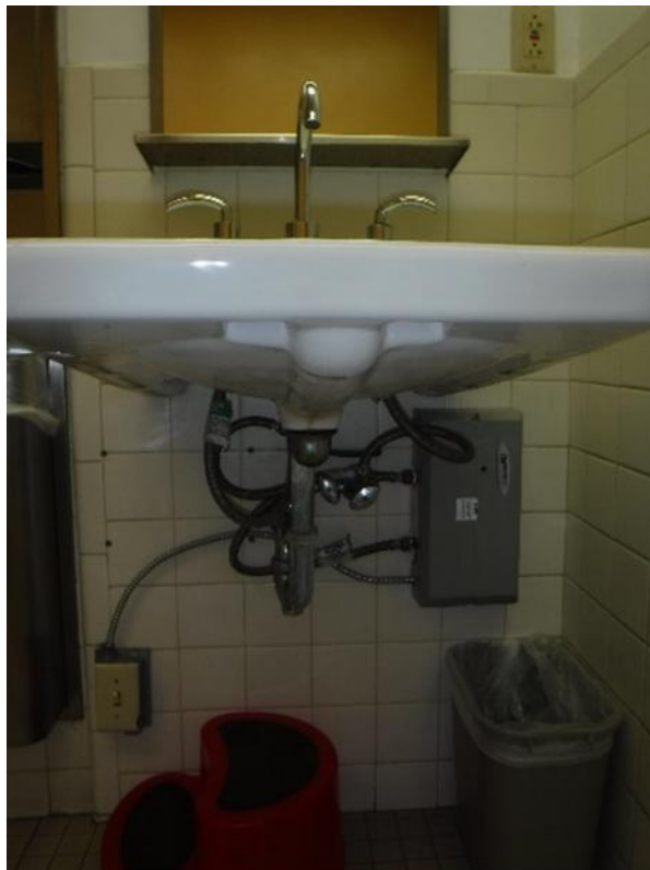
Lobby Restroom Tankless Electric Water Heater
