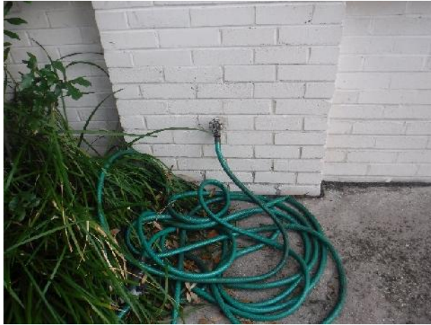
Exterior Wall Mounted Hose Bibb
