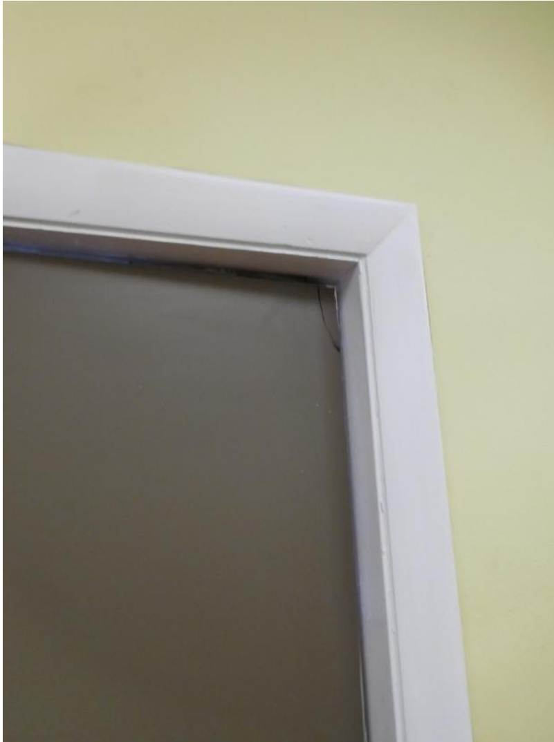
Damaged Staff Room Door
