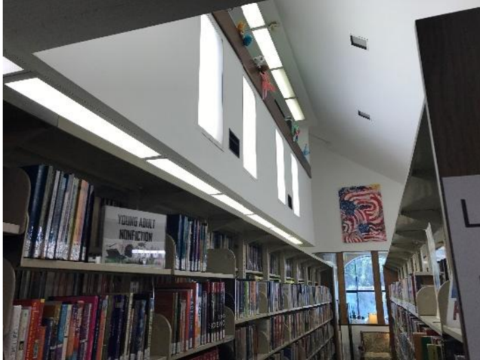
Supply Air Diffusers at Reading Room
