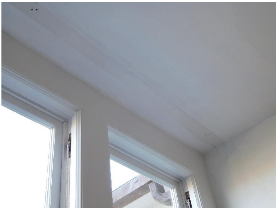
Adult Reading Room wood window system; note water damage
