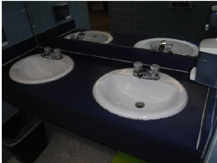
1 st Floor Women's Restroom Lavatories
