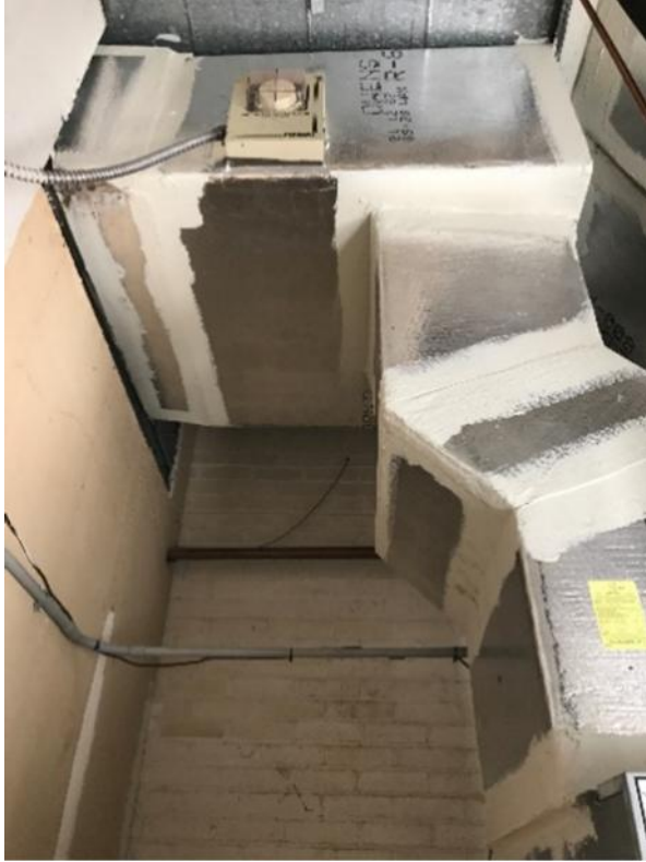
Fiberglass Ductwork at Mechanical Room
