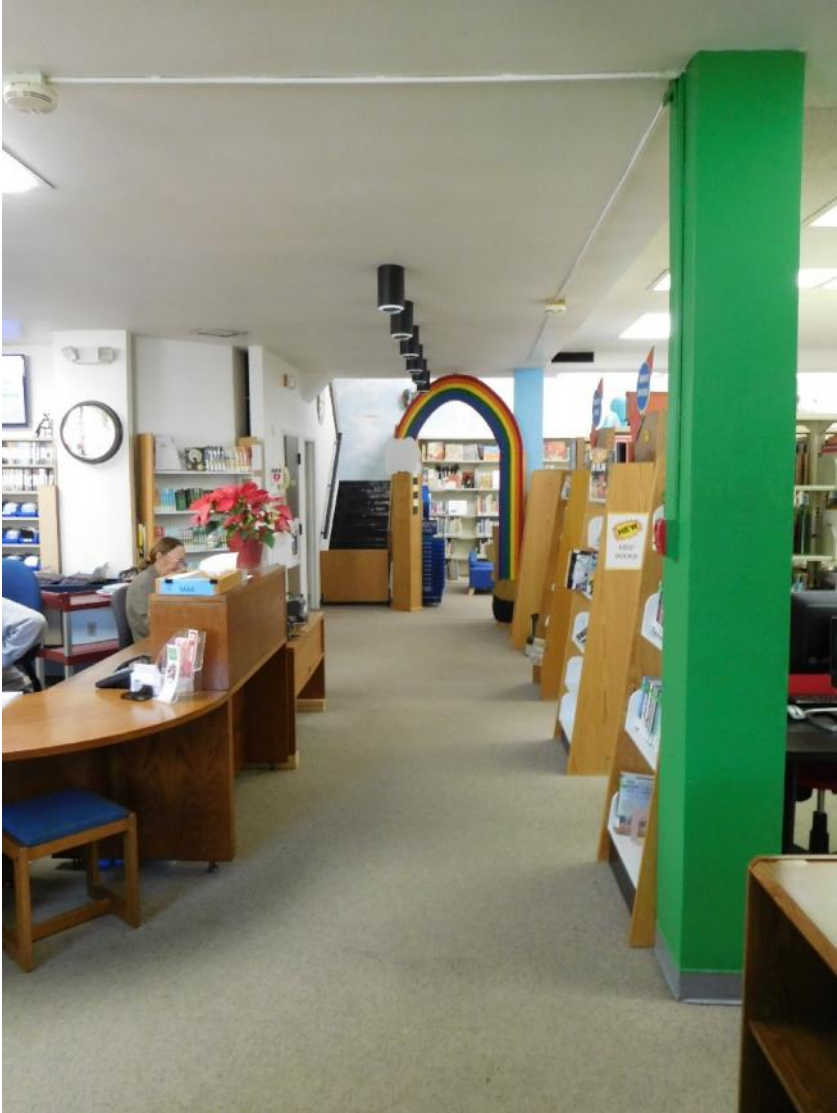
Note exposed electrical conduit in Main Library
