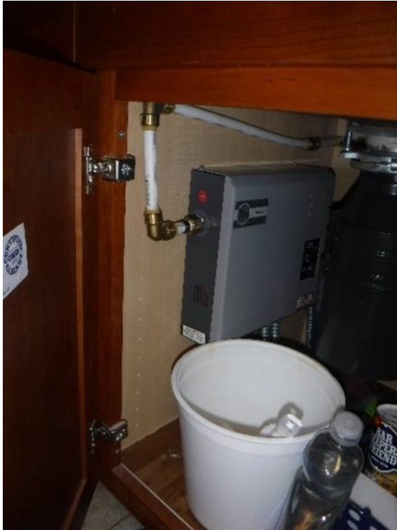
First Floor Multipurpose Break Room Electric Water Heater
