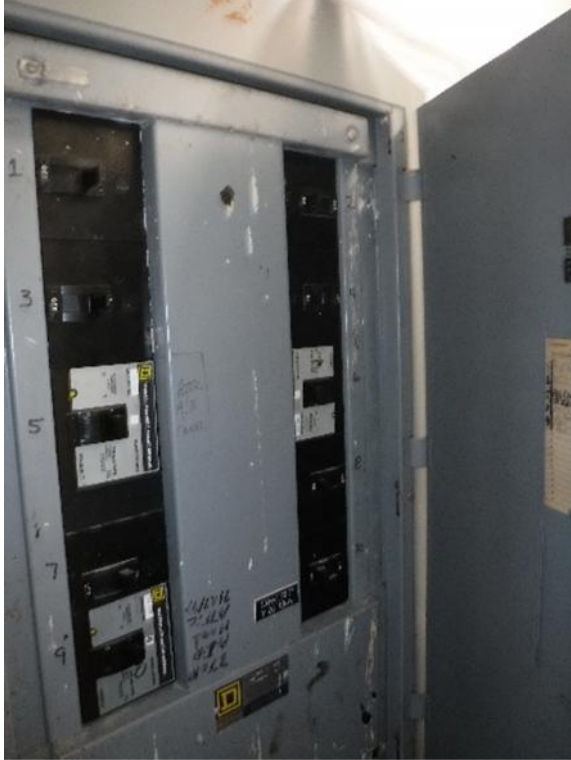
Main Distribution Panel
