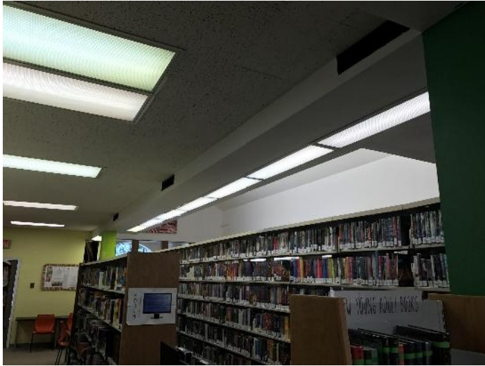
Supply Air Diffusers at Reading Room
