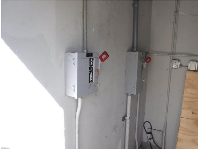
Interior Disconnect Switches
