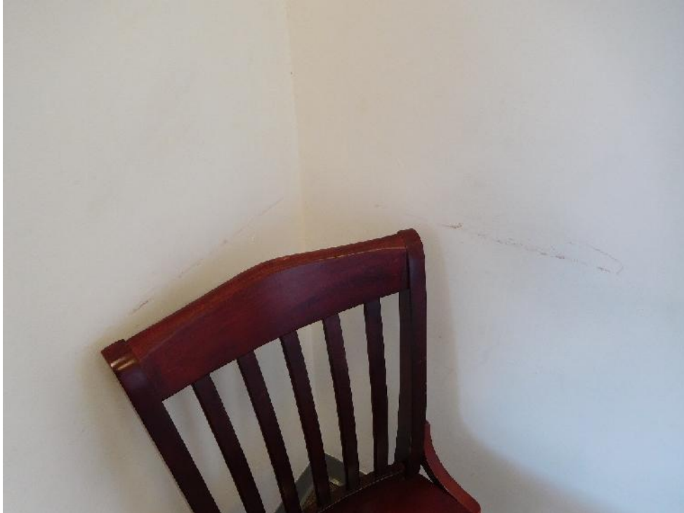
Chair scuffing of wall surface
