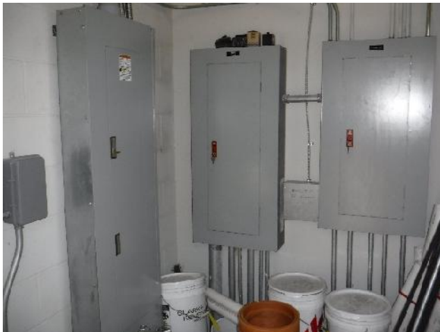
Main Electrical Room Distribution Panels
