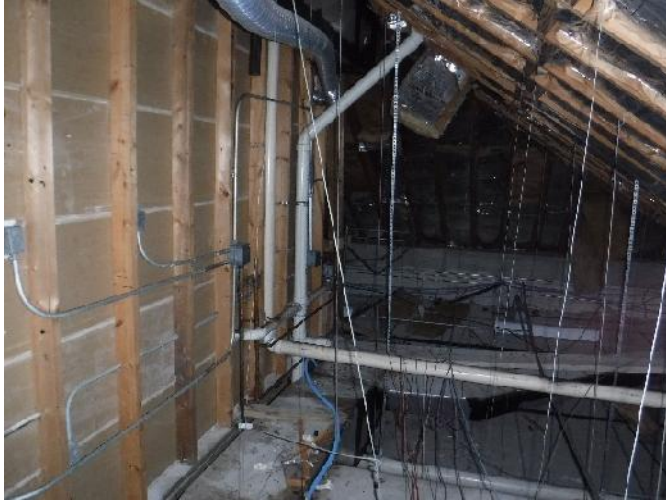
Domestic Water Plumbing Piping
