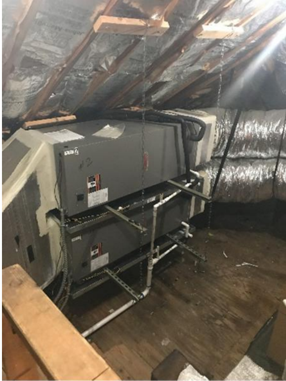
(2) 5 Ton Air Handling Units
