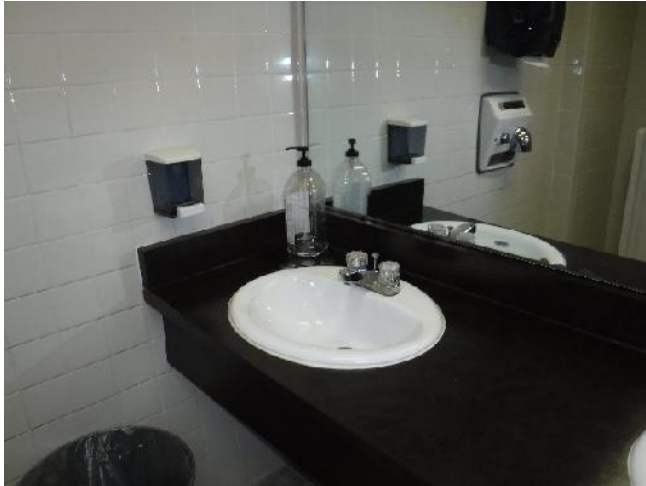
1 st Floor Men's Restroom Lavatories
