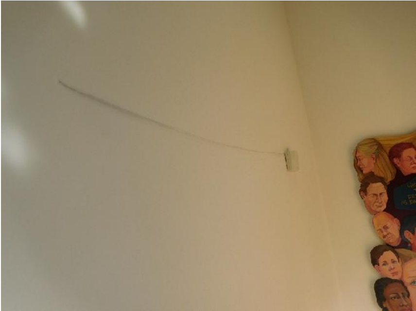
Adult Reading Room; exposed electrical lines
