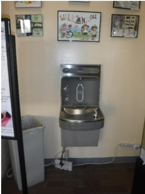
Lobby Electric Water Cooler
