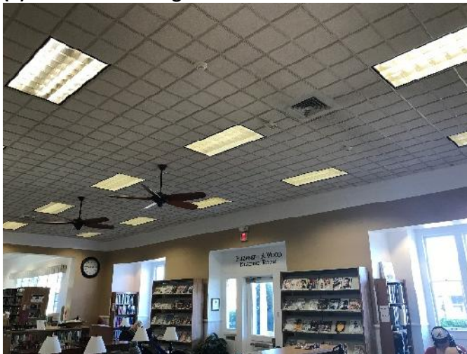
Supply Air Diffusers at Reading Room
