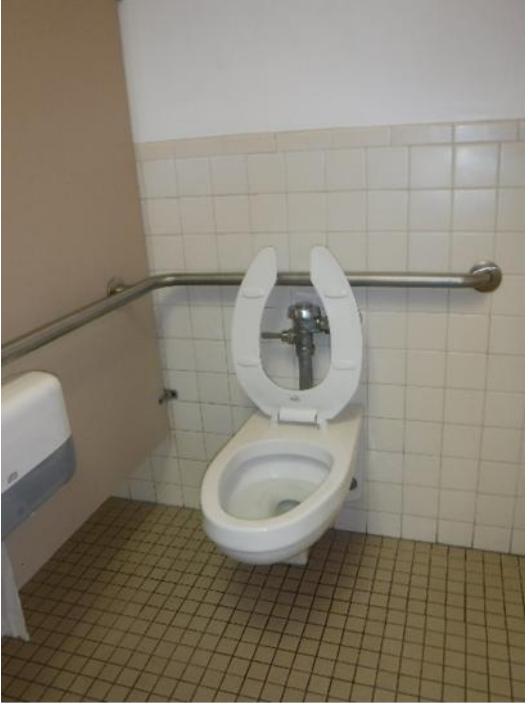
Lobby Men's Restroom Water Closet
