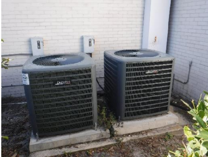
(2) 5 Ton Condensing Units
