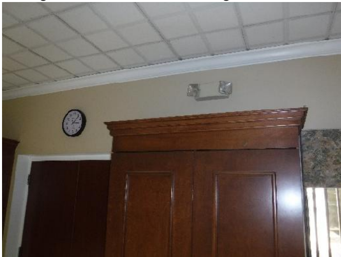
Typical Emergency Lighting
