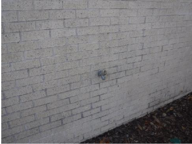
Exterior Wall Mounted Hose Bibb
