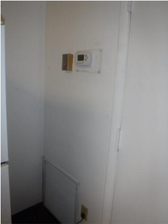
Return Air Grille & Thermostat (AHU-2.1)
