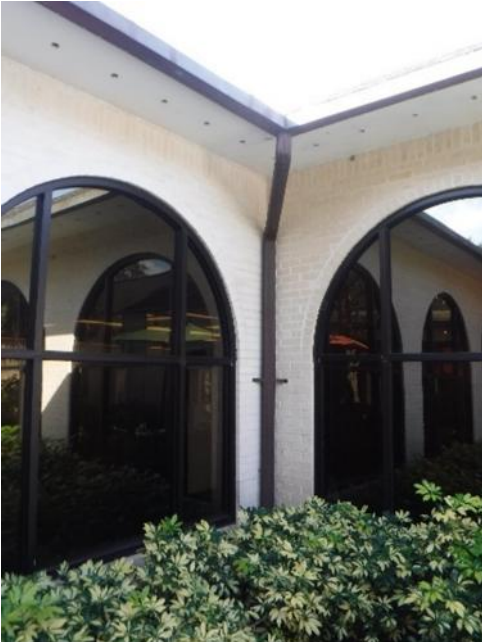
Gutter and Downspout Storm Drain System
