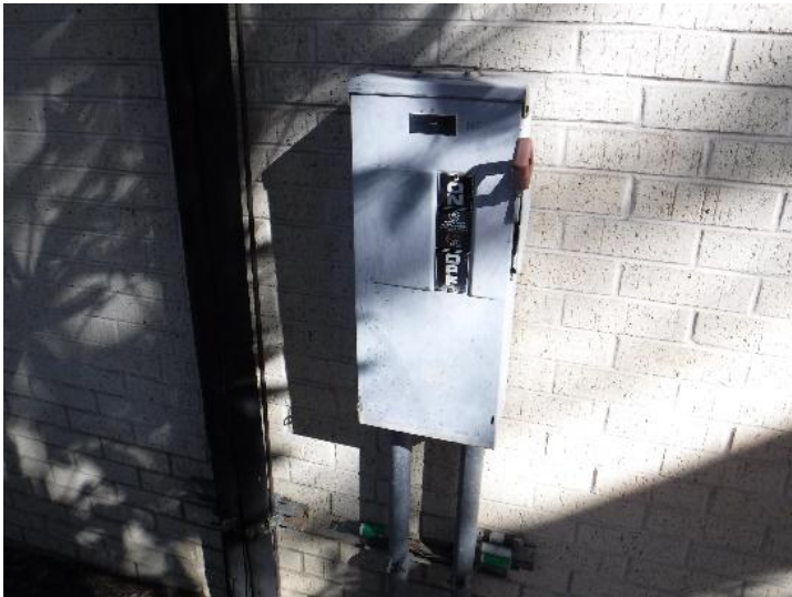
Exterior Disconnect Switch
