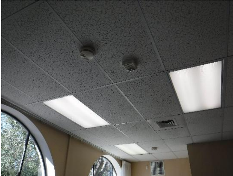
Typical Notification Device and Smoke Detectors
