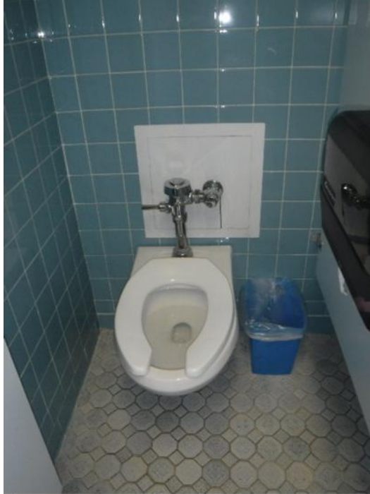
1 st Floor Women's Restroom Water Closet
