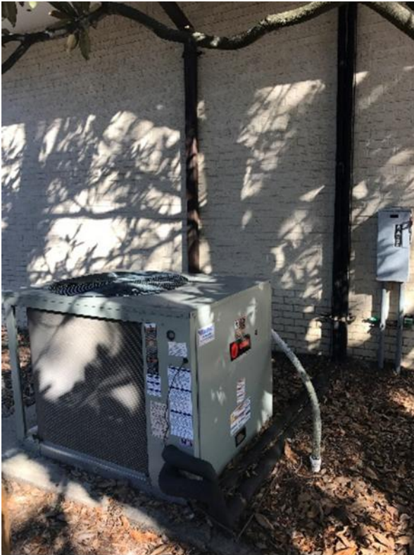
10 Ton Condensing Unit (CU-3)
