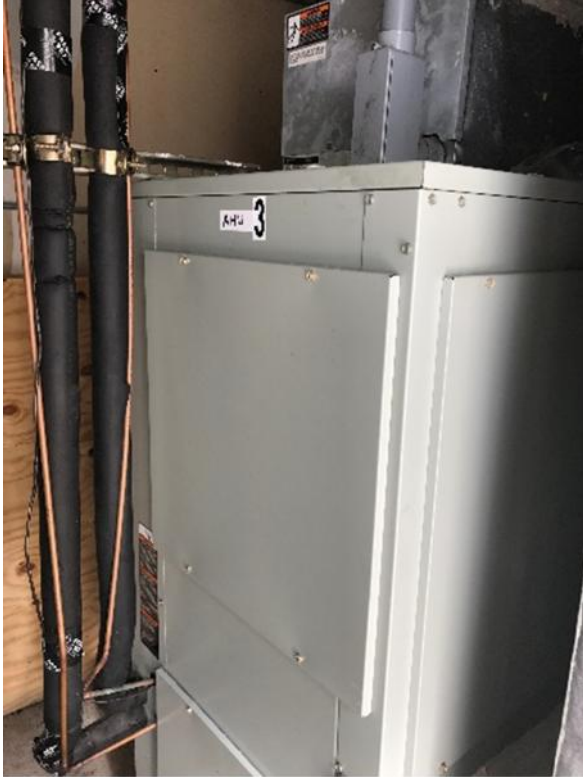
10 Ton Air Handling Unit (AHU-3)
