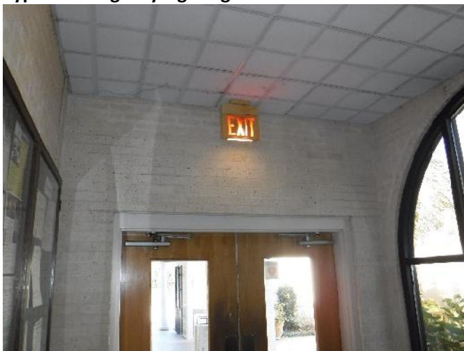
Typical Exit Sign
