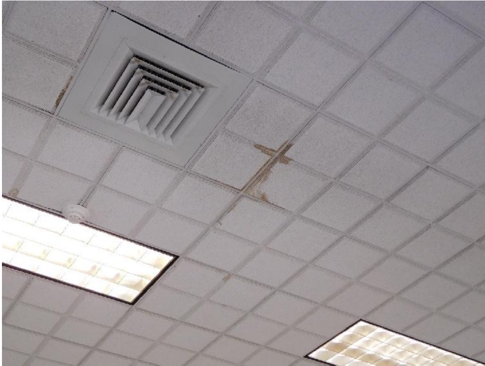
Water stain of ceiling tiles
