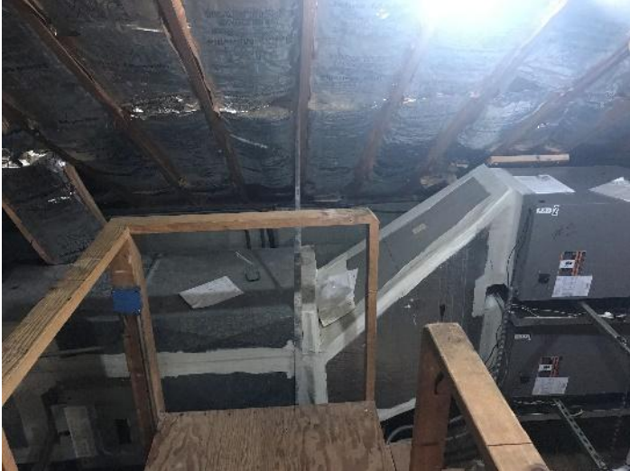
Fiberglass Supply Air Ductwork at Mechanical Room
