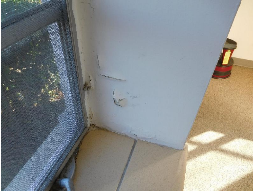
Adult Reading Room; note water damage
