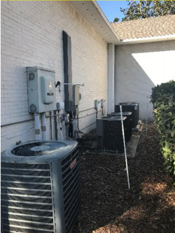
3.5 Ton Condensing Unit (CU-2.1)
