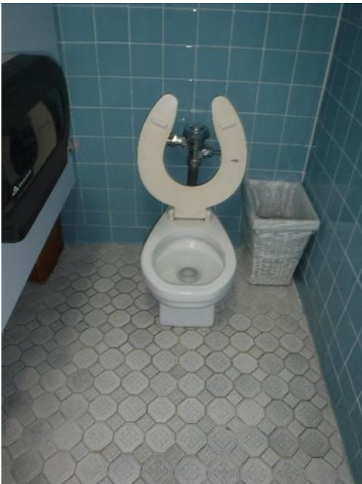
1 st Floor Women's Restroom Children's Water Closet
