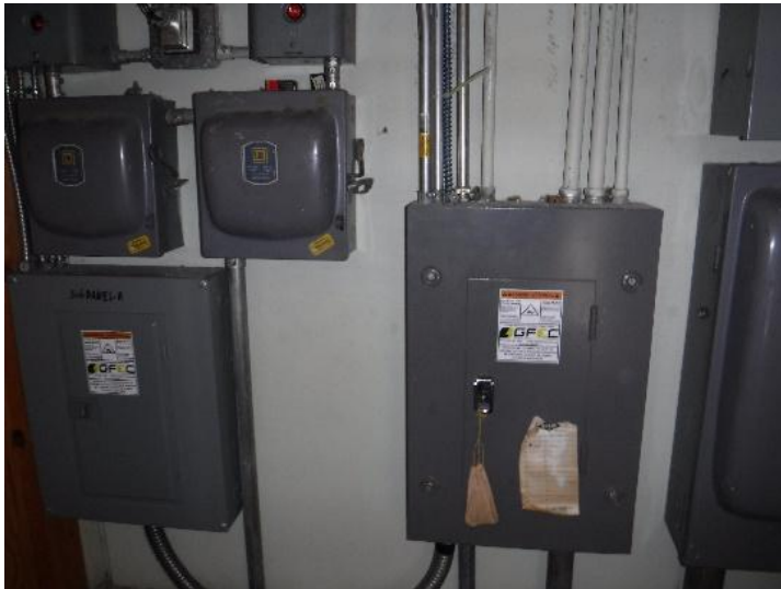
Electrical Closet Sub-Panels
