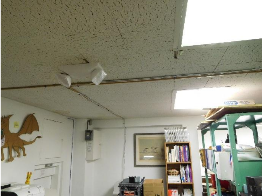
Mezzanine; exposed electrical lines
