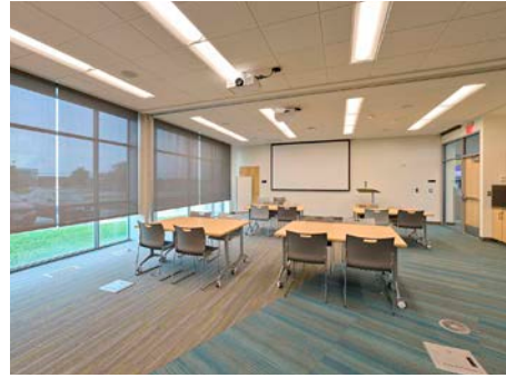
Motorized window shades to control sunlight
